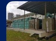
Odour Scrubber System
